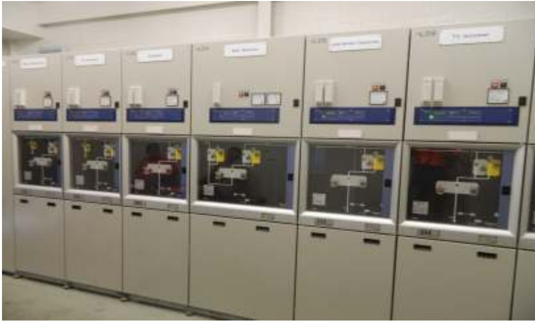
Switchgear inside the Salelologa Substation
