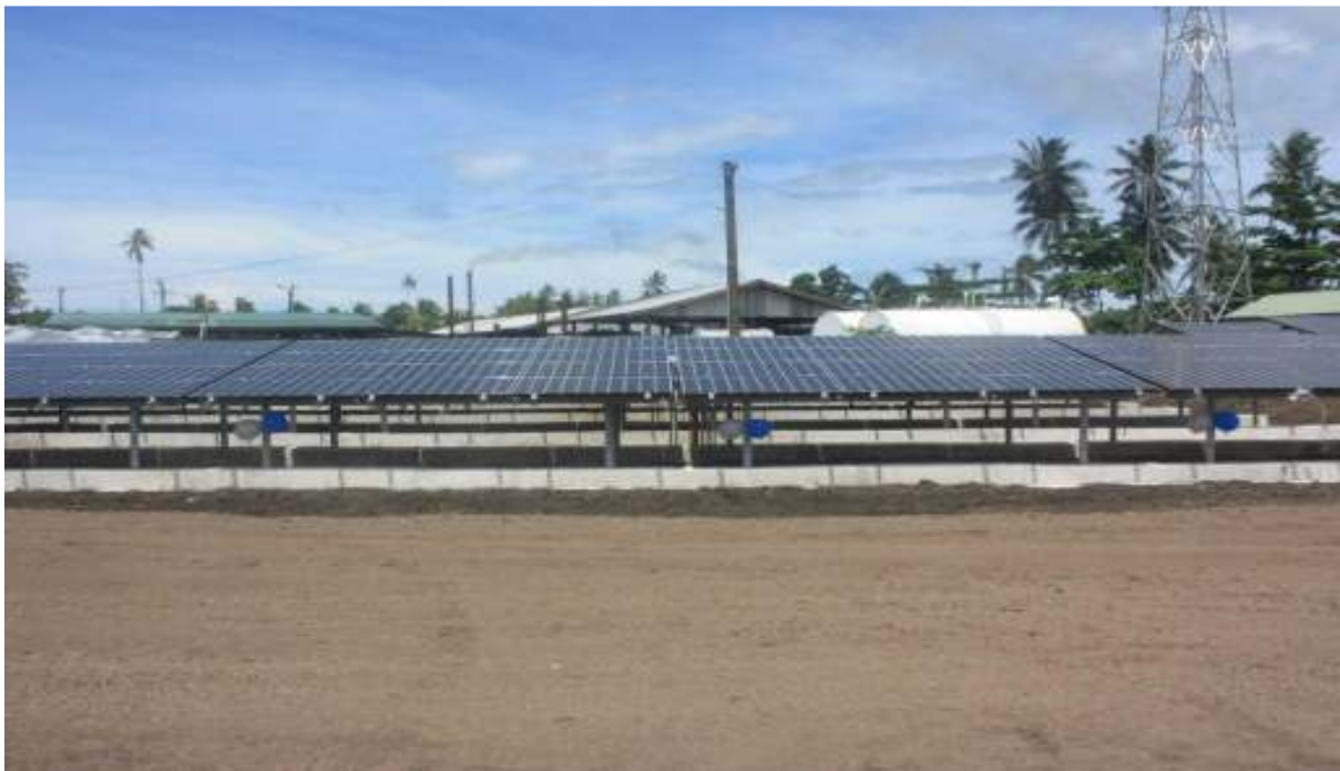
Front view of the Solar farm
