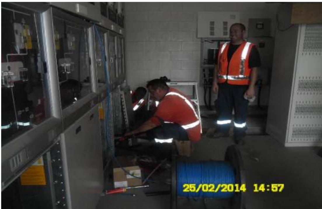
Northpower technicians Russell Jamieson and Stuart Reid at work at the Salelologa Substation
